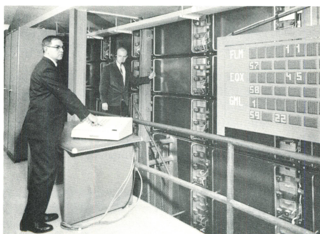
A view of the control area behind the display boards with a test keyboard in the foreground and the dual control system in the rear.
