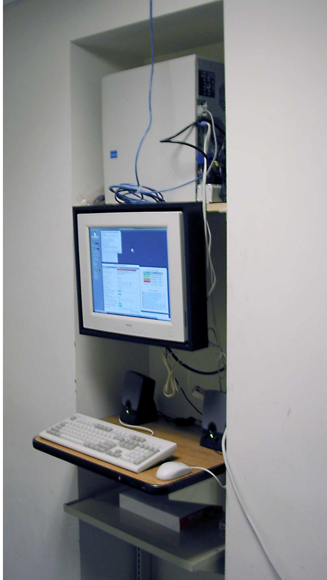
Figure 3-8: MoreMagic Network and Server Diagnostic Console Kiosk
