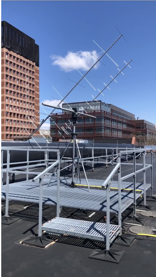
(a) Antenna Site
